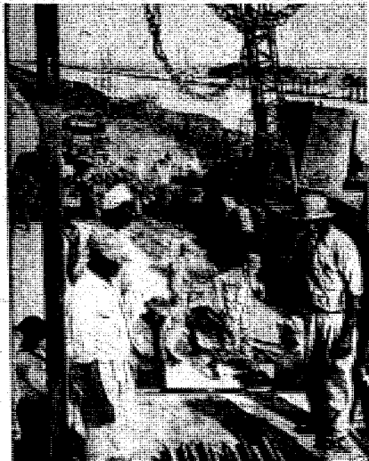
GETTING READY TO WORK —The 78th Engineers and a group of Florida volunteers get construction of a pontoon bridge under way near Belle Glade, Fla.
