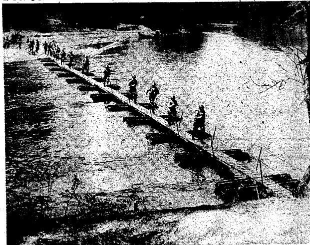
ON THE DOUBLE, SOLDIER —Seven minutes after the first section of bridge is "water borne," 150 feet of bridge is in place and the first troops are on their way across the Upatoi creek.
